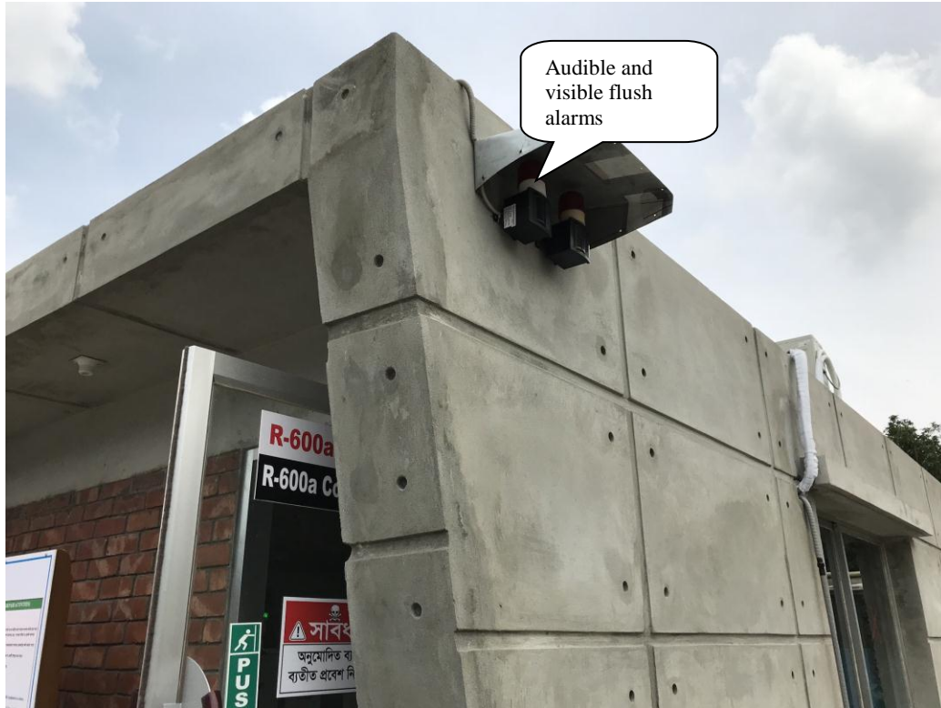
Figure 4.4: Control Room for Storage Tank including visible and audible alarm outside
