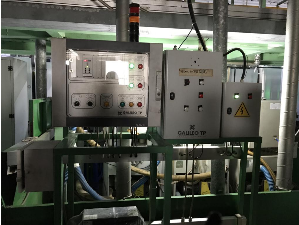
Fig. 4.6: R600a Charging Stations with visible and audible alarms.
